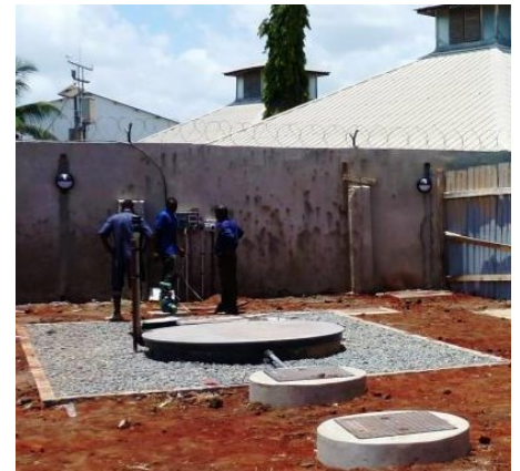
Mars 5000 installed in Tanzania
